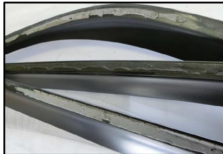
Double-Sided Tape in Bad Condition
